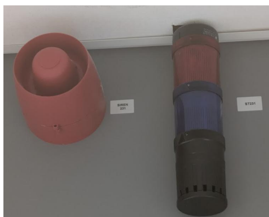
Figure 3: Alarm indicator. These are in several locations within the MST-Lab infrastructure.
